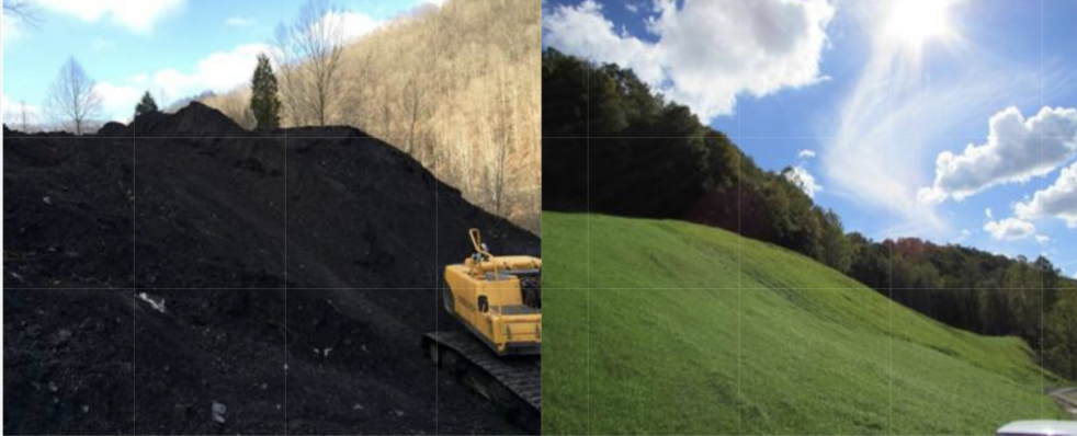
A slope of the Hurricane Creek GOB Pile during extraction and cleanup, and the remediated site after reclamation. Source: Dominion Energy
